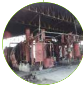
Tyre Pyrolysis Plant Ratlam, Madhya Pradesh
